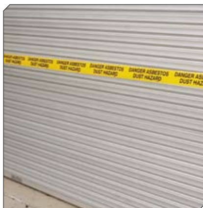
Figure 3: Barrier formed using tape (appropriate for small non-friable removal jobs or as part of system using other barriers such as hoarding).
